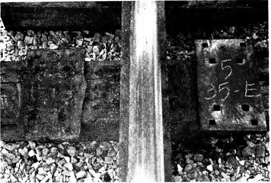
Fig. 20. South Portion Section 5. 13-in Bird 7-ply Duck-Felt Tie Pad, Coated, After 83-months' Service in the Inner Rail of the Long 4-1/2° Curve
